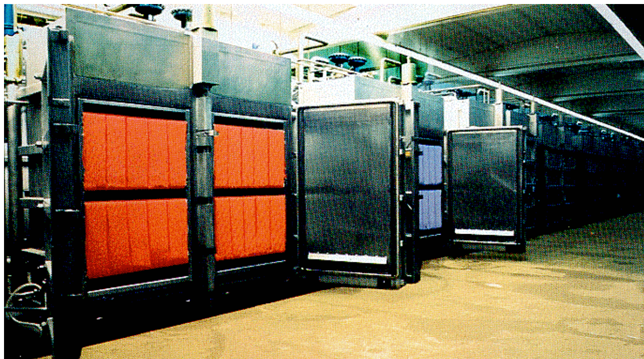
Large hank dyeing plant for knitting yarns with automatic liquor preparation tanks and kitchens.
