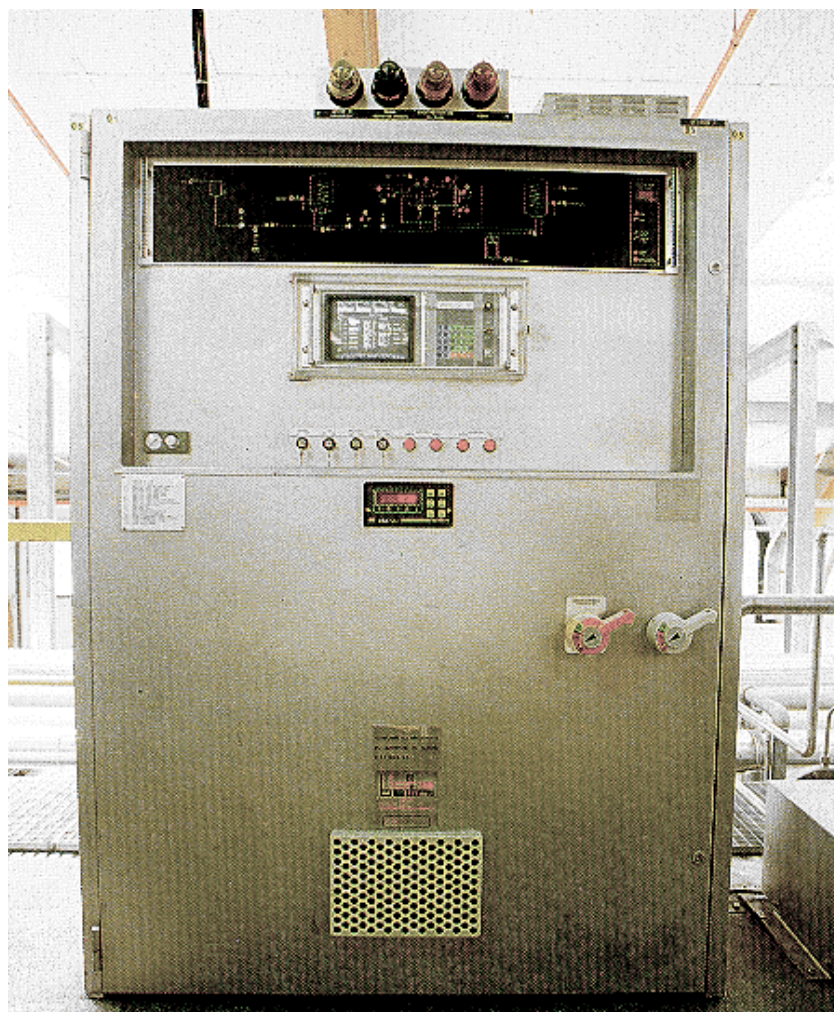
Electric control panel with microprocessor for automated drying cycle control on ARSPO pressure dryer.
